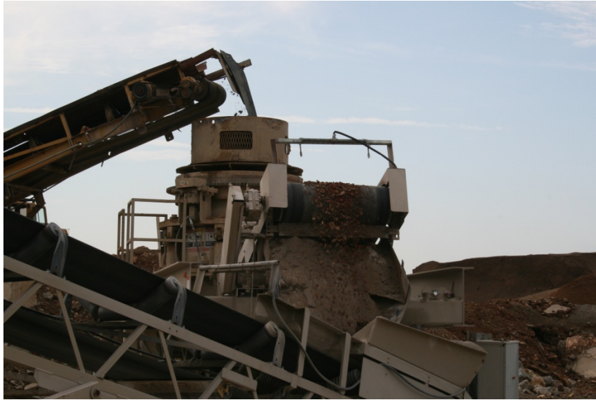
Figure 3-5: Rotary crusher apparatus at D.H. Griffin Crushing and Grading.
