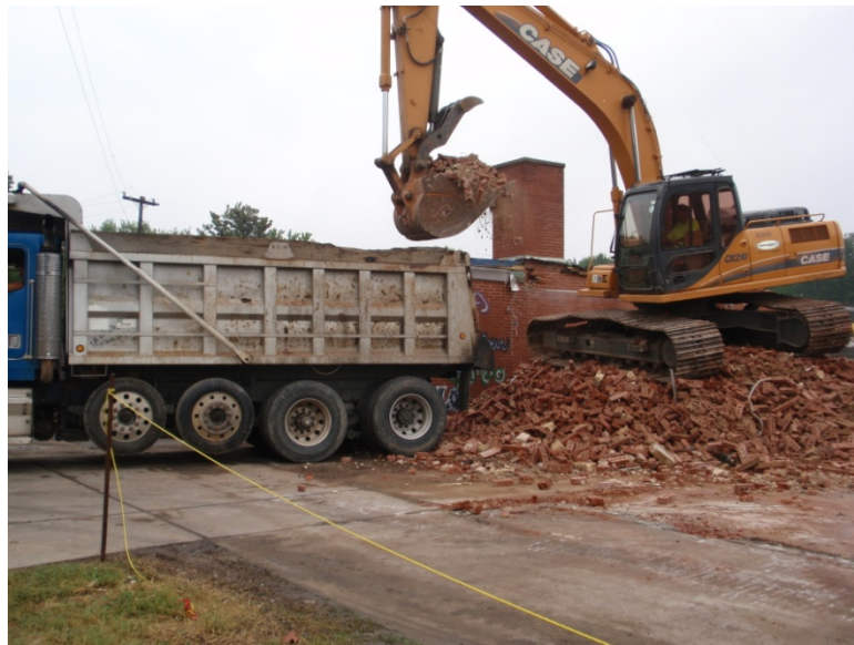
Figure 3-3: Demolished brick masonry from Idlewild Elementary School, loaded into a separate dumptruck for transport to D.H. Griffin Crushing and Grading.
