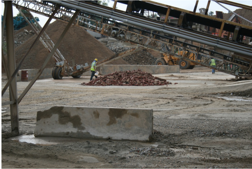
Figure 3-4: Demolished brick masonry from Idlewild Elementary School, stockpiled at D.H. Griffin Crushing and Grading, prior to being crushed into aggregate.
