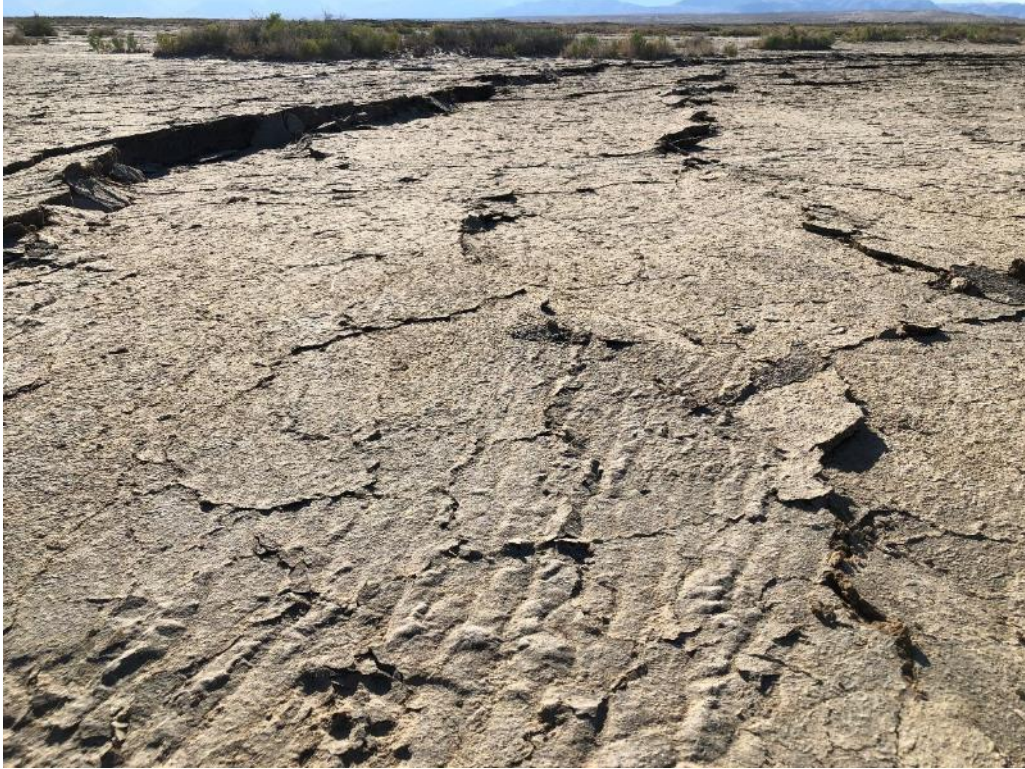
Figure S1. Lateral spread features in the Paxton Ranch area on 7/10/2019. Curved, discontinuous zone of disturbed lateral spread cracks with vertical displacement, and some compressional cracks. Lat. 35.809808°, Lon. -117.634767°. Photo 8331 credit B. Olson, CGS.
