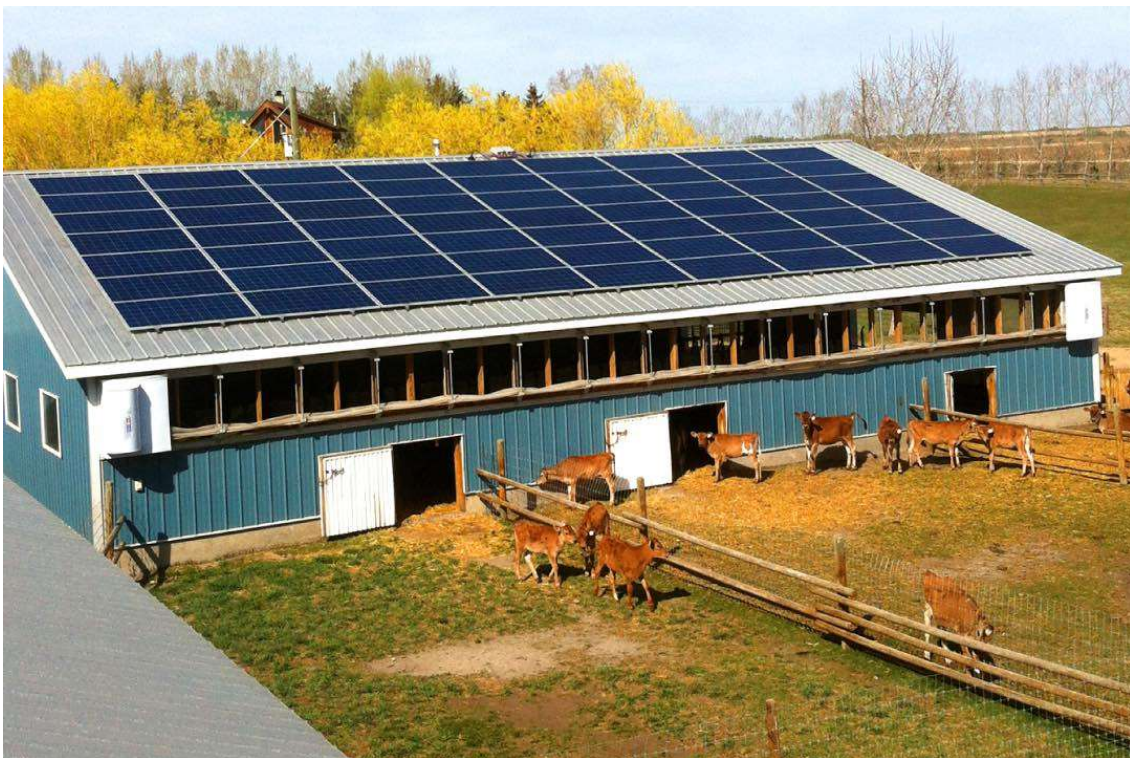
Figure 3-9: A calf shed using solar panels as a source of electricity (source: www.skyfireenergy.com )
