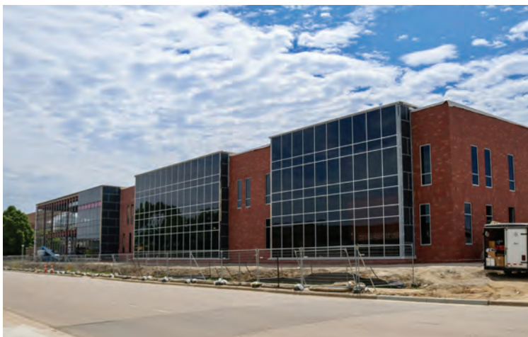
Above: Construction progress of the Raven Precision Agriculture Center on the SDSU campus as of June 5.
