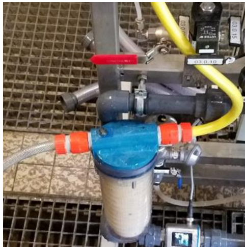
Figure 2-3 Filter for Secondary Effluent
