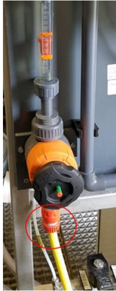
Figure 2-4 Inlet Feed Water Attached to Installation
