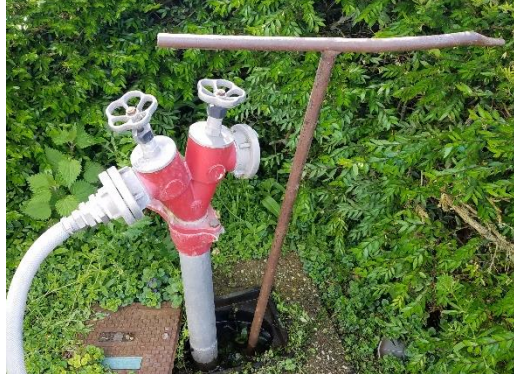
Figure 2-1 Hydrant for Secondary Effluent
