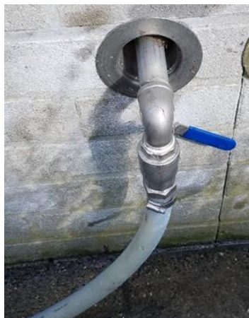
Figure 2-2 Valve for Secondary Effluent
