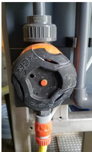
Figure 3-1 Dial for Influent Flow into Pilot System
