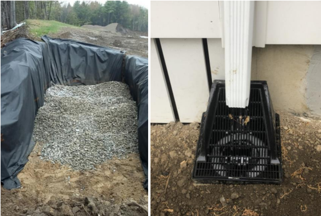
Figure 4.10: Infiltration Trench for Residential Rooftop (left) and Downspout with Self-Cleaning Grate (right)
