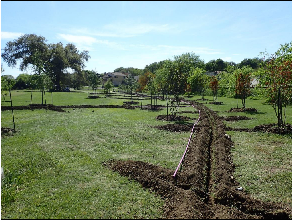
Figure 8. Overview of Irrigation Lines within 41BX1799, camera facing southwest
