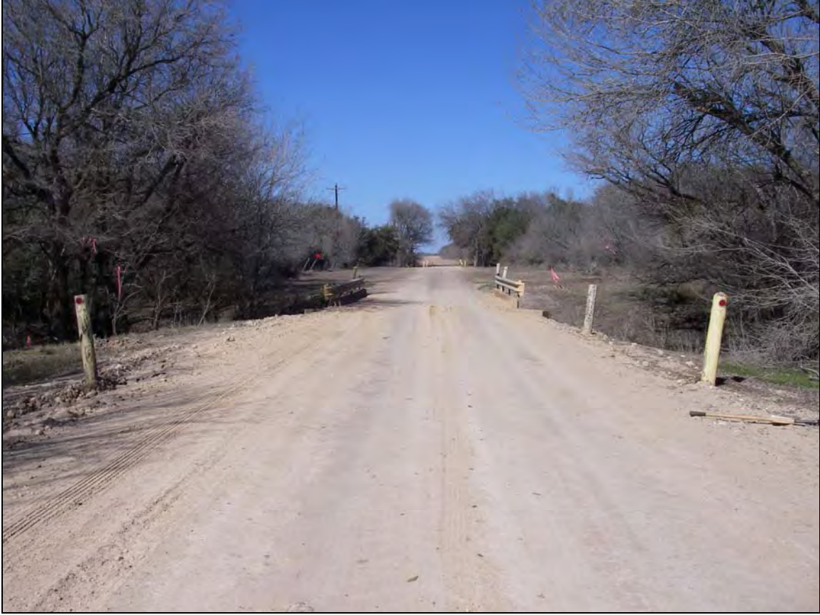
Figure 9. Overview of Peck-Bush Road and graded imported road fill near the southern Peck-Bush Road at San Miguel Creek crossing, facing north.
