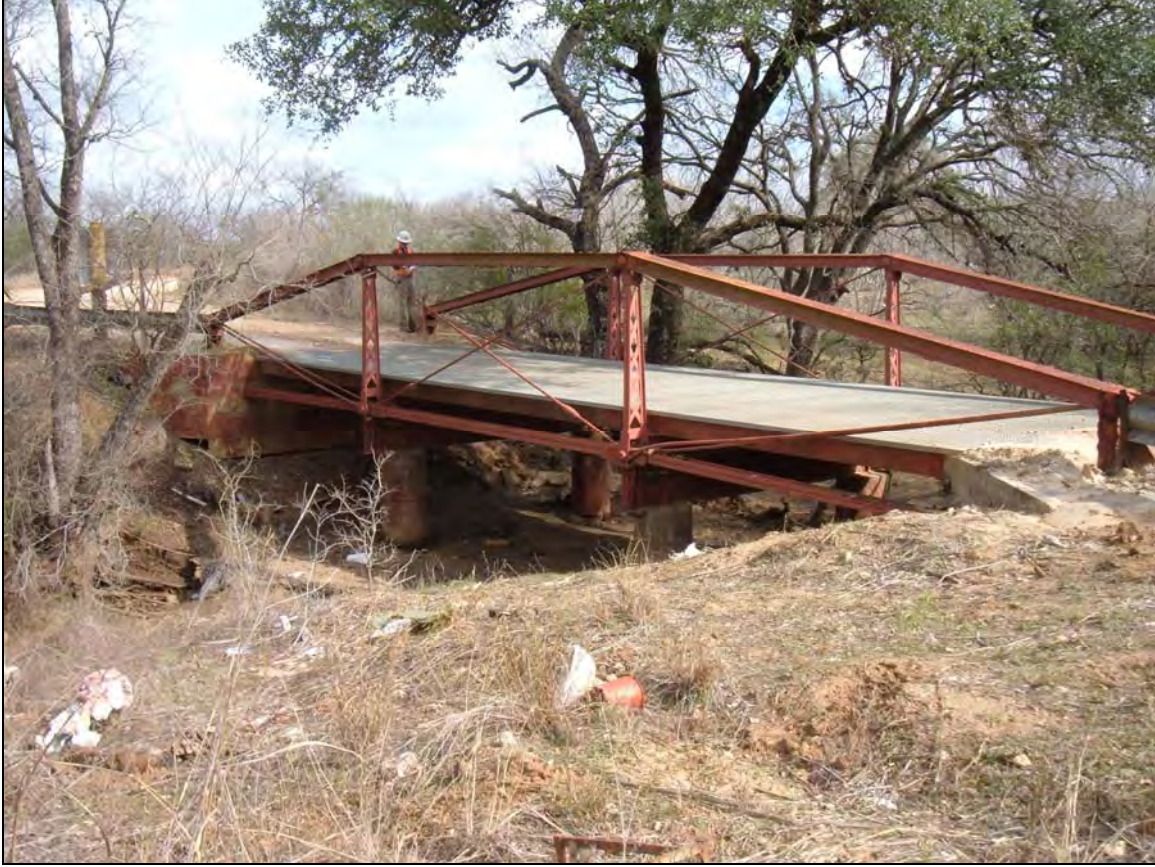
Figure 13. Overview of the Andy Sadler Road at Live Oak Creek bridge, facing east/northeast.
