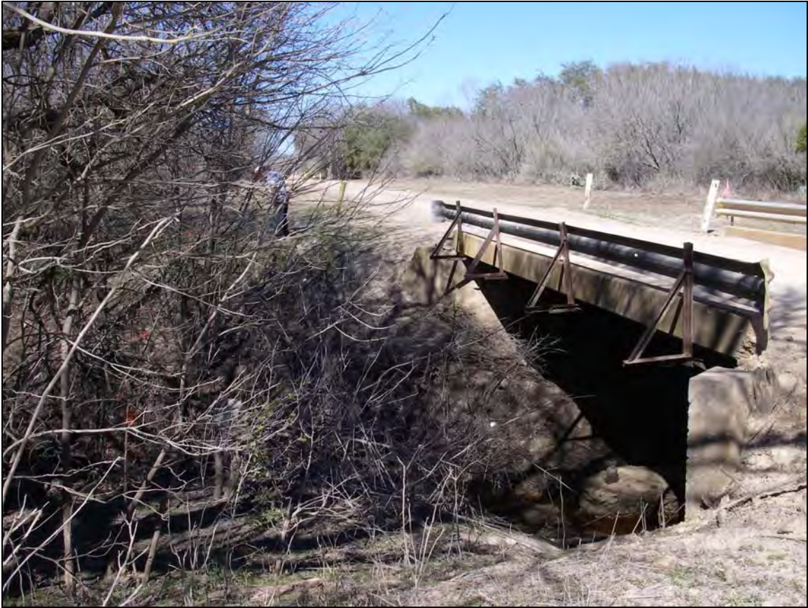
Figure 5. Overview of the bridge over the southern San Miguel Creek divergence at the Peck-Bush Road crossing, facing northeast.
