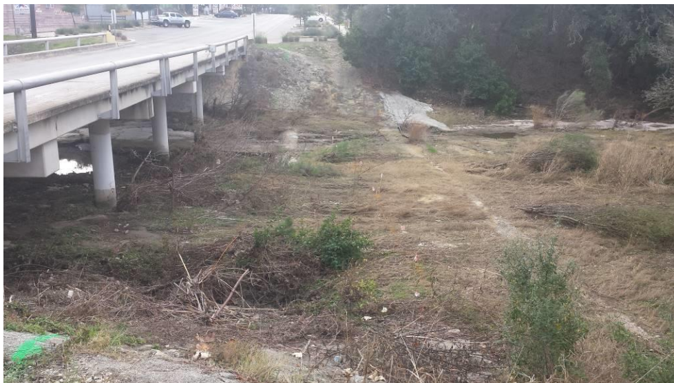
Photo #12: View south across Helotes Creek at the location of the proposed pedestrian bridge. Note the linear concrete features marking buried utility lines.
