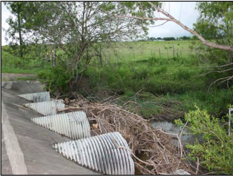
Figure 8. Overview of cutbank on upstream side of crossing; facing southwest.
