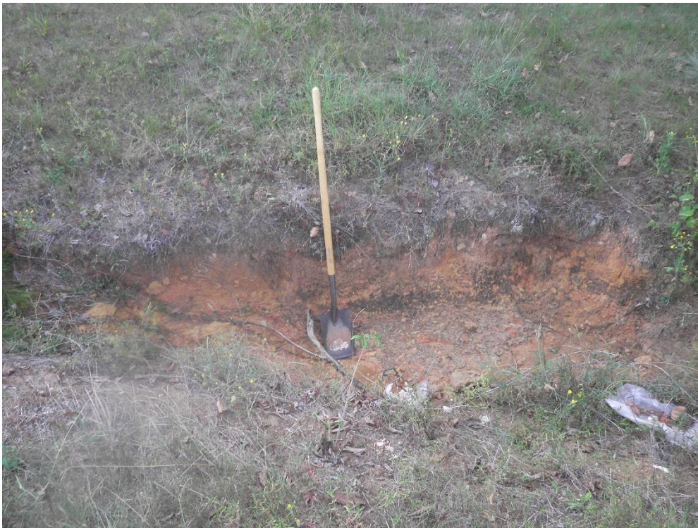
Figure 6. Example of an erosional blow-out along the existing roadway; south is toward the top of the photo.
