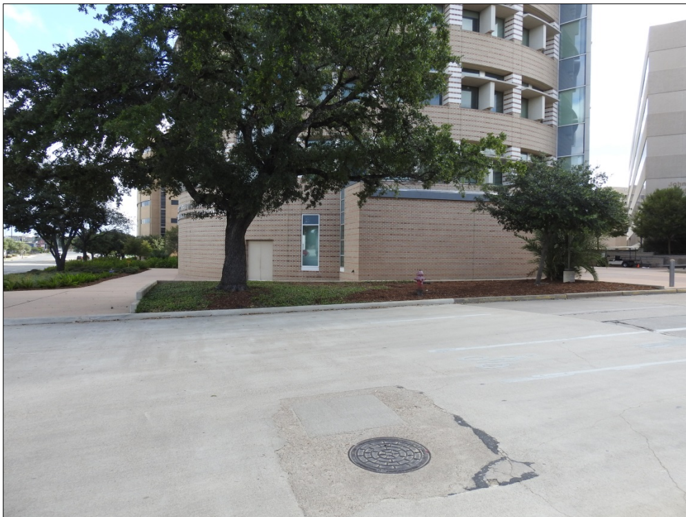
Figure 4-7. Pavement, Sewer Line, and Water Line on South Side of University Drive, Facing Northeast.
