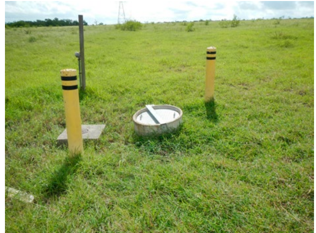
Figure 6.80. Modern water meter on 41GU176.
