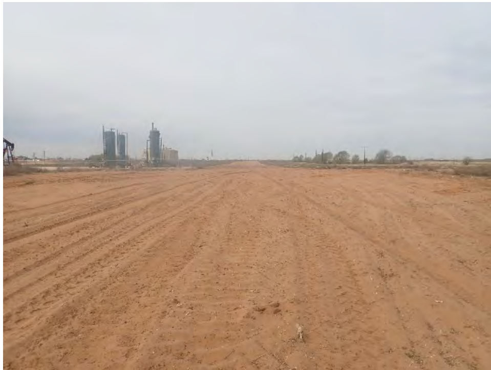
Figure 5-9. Overview of active pipeline work taking place within the southern half of Site 41MD58 at the time of delineation survey. View is to the east.
