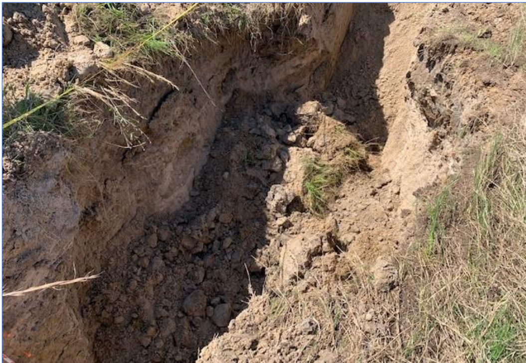
Figure A-6. Overview of Collapsed THT-2 (Facing North)
