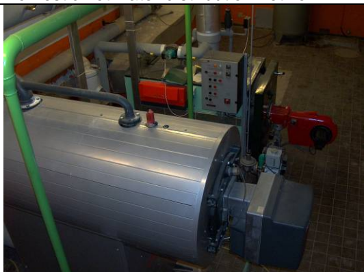
Boilers, condensing and traditional.
