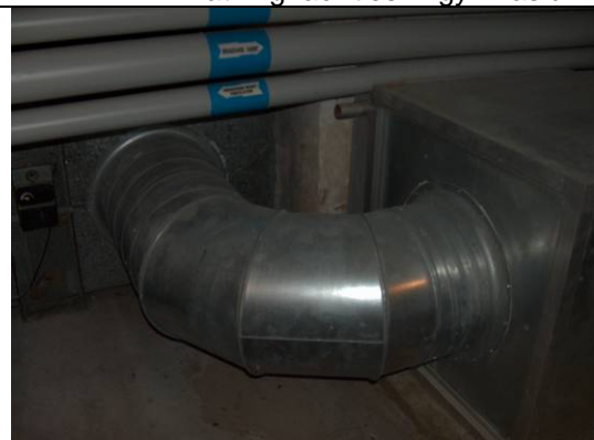
New, un-insulated ventilation system.
