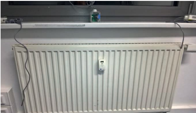
Figure 4: Measurement points at radiators
