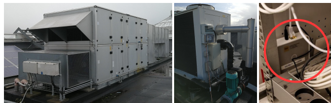
Fig. 1. From left; AHU, chiller unit and Building Management System (BMS) gateway for remote data acquisition and control, situated at Kolding Storcenter, a Danish shopping center.
