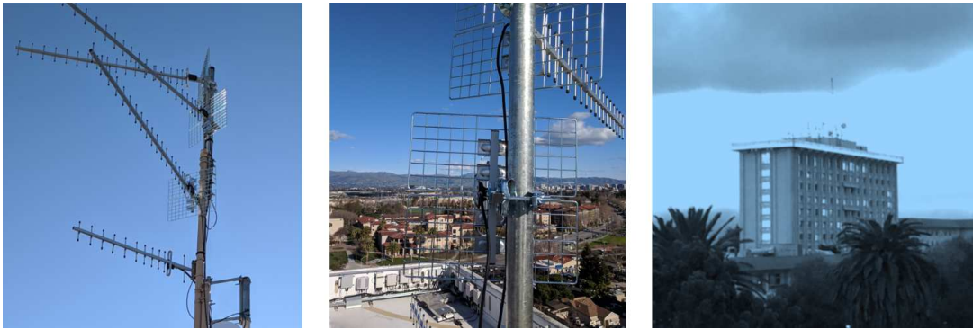
Fig. 4.2: Four directional antennas connected to the Gateway. The Gateway has been installed on top of a 11-level building in Santa Clara.
