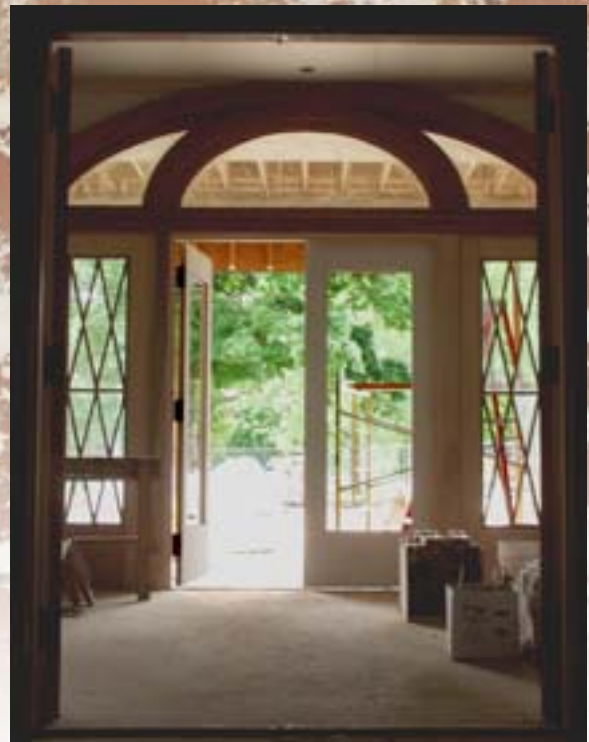
Interior renovations are restoring Carnall Hall's architectural finery. The overhaul will give the former women's dormitory new life as a hotel and restaurant.
