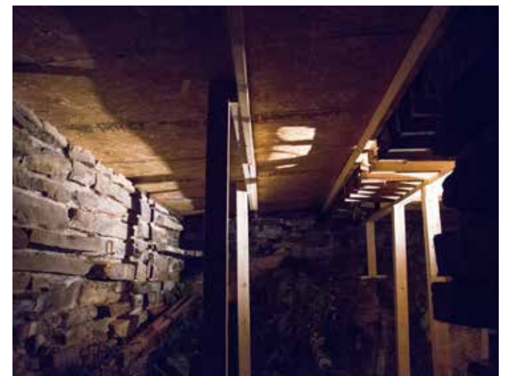
Middle, Fay Jones' home office studio on the home's ground level. Above, repairs to supports on the home's ground level. (Photos by Russell Cothren)
