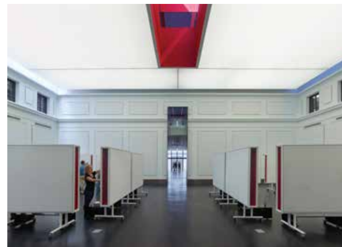
A fabric dropped ceiling conceals the nearly 400 fluorescent tubes that provide lighting for the second floor gallery of Vol Walker Hall.
