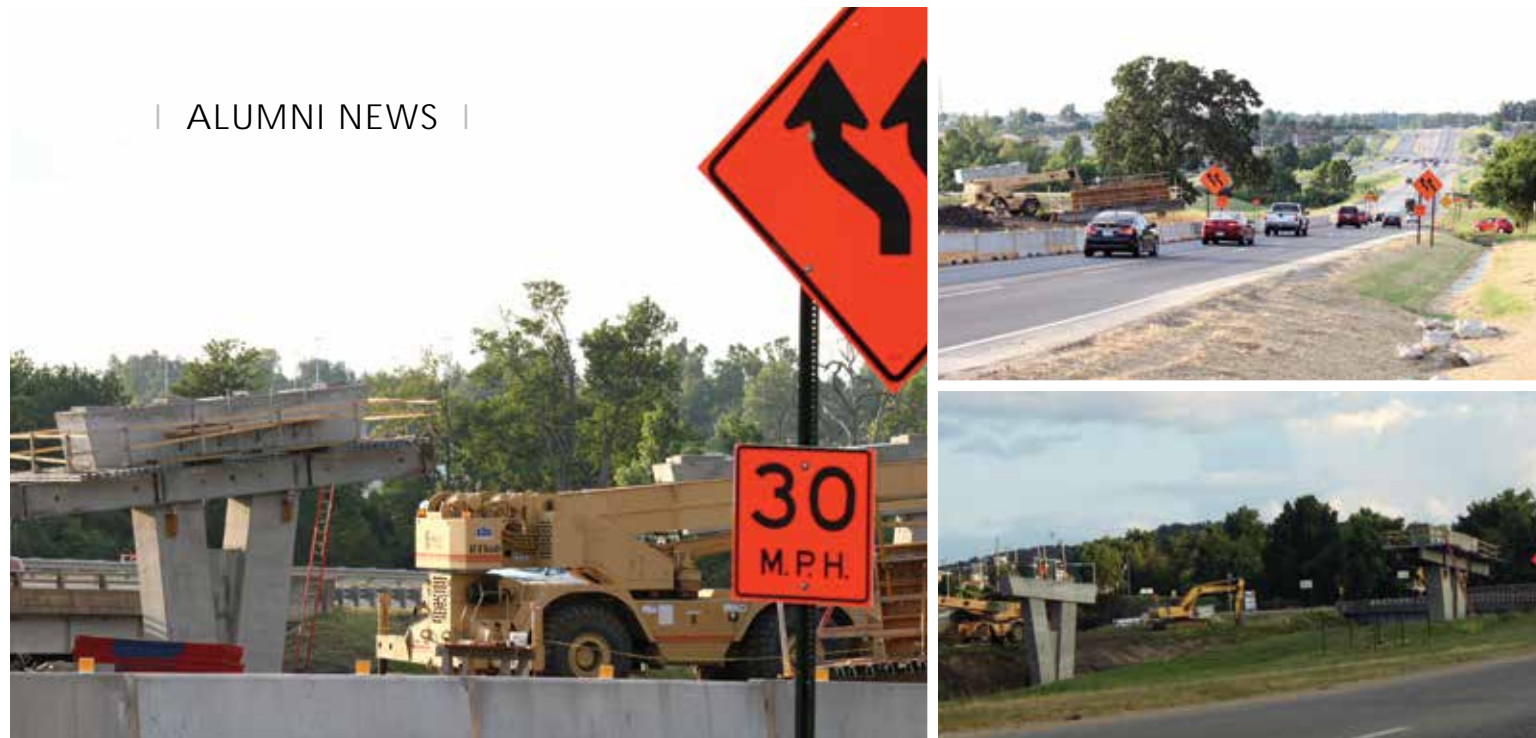
The flyover bridge in north Fayetteville will provide direct access from College Avenue to I-540, so northbound drivers don't have to make a U-turn at the Joyce Boulevard traffic light. Construction could continue until early 2015.
