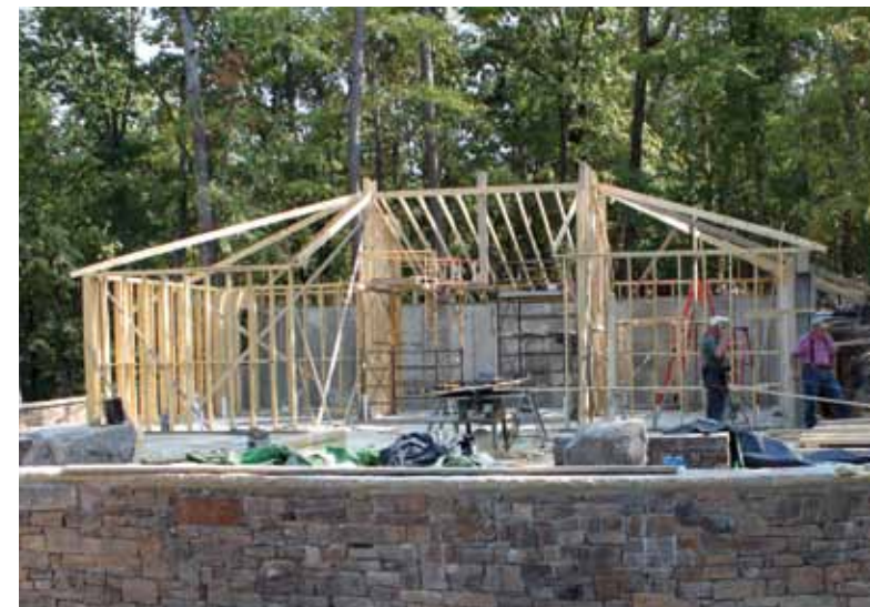
Stuart Perry, left, and Mike Brown, construction supervisor at the gardens, work on a building at the Perry Wildflower Meadow Overlook in September 2010.
