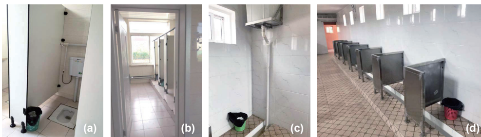
Figure 1. Sanitation facilities of each school. (a) (b) School A toilet, (c) (d) School B toilet. (Taken by the author)
