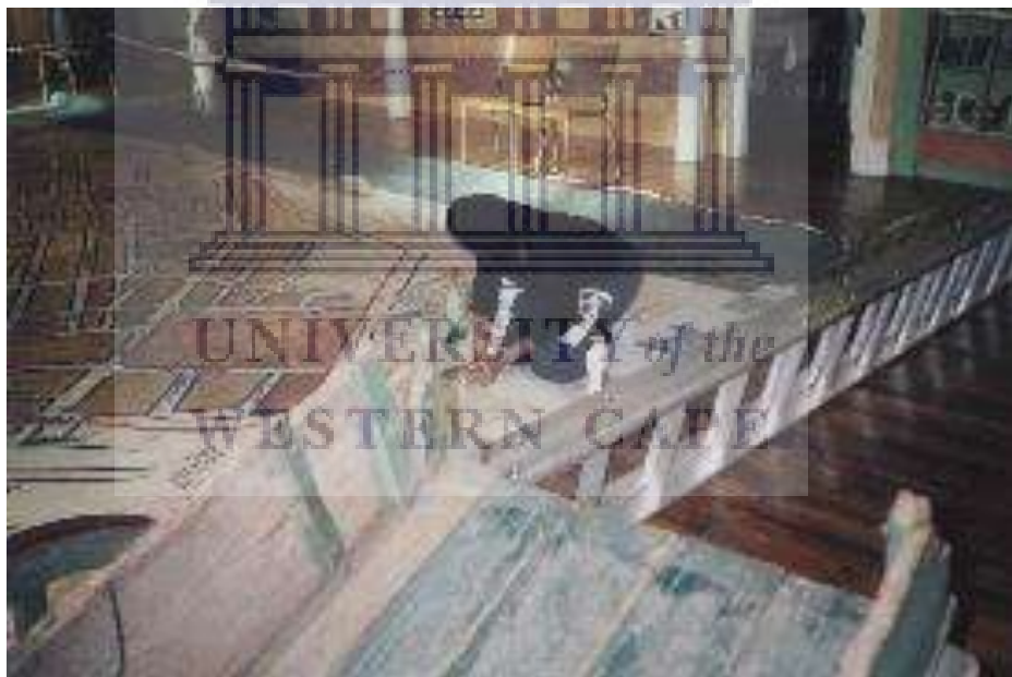
Figure 2.15: Installing District Six painted floor map with a plastic overlay with the District Six hawkers' barrow in the foreground. Digging Deeper exhibition. Photograph: D6M archive.
