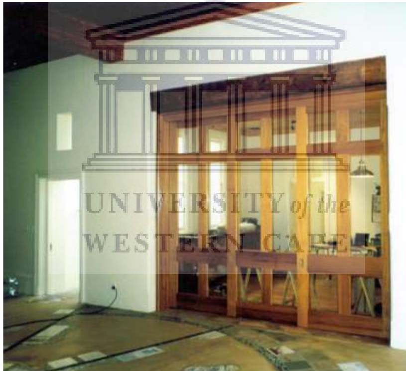
Figure 4.20: Walls opened up and doors installed to create a District Six Museum coffee shop open plan design in the District Six Museum memorial hall. Photographs: Rennie Scurr Architects.
