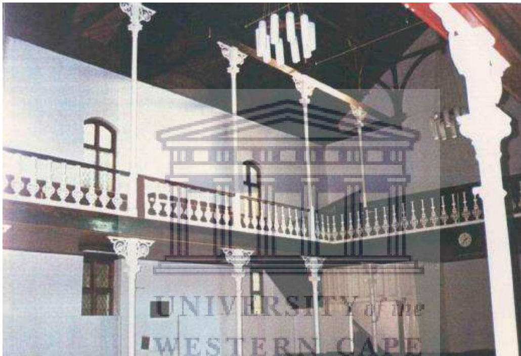
Figure 4.8: Buitenkant Methodist Church interior view of the upper gallery from below 1993. Photograph: Rennie & Goddard Architects.
