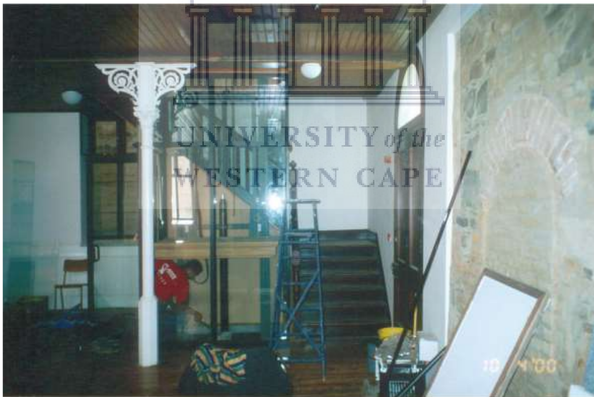
Figure 4.22: Installation of the District Six Museum lift for disabled visitors. Note older warehouse material fabric to the right-left exposed to form part of the Digging Deeper exhibition 10.04.2000. Photograph: Rennie & Scurr Architects.
