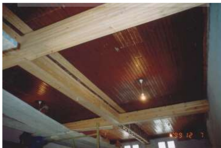
Figure 4.19: Stepping Stones classroom and entrance were reconfigured as the District Six Museum Memorial Hall. Columns were removed and I beams installed to support the ceiling to provide an open plan design. Photographs Rennie Scurr Architects.
