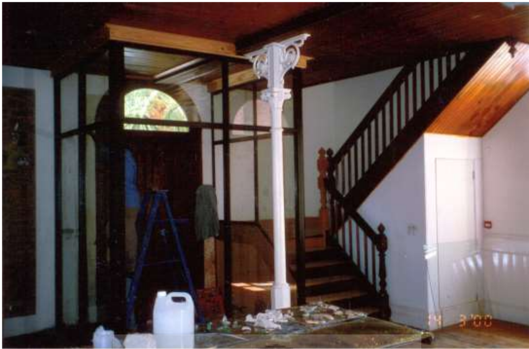
Figure 4.21: Installation of the District Six Museum black aluminum and glass entrance lobby, 14.03.2000. Photograph: Rennie & Scurr Architects.
