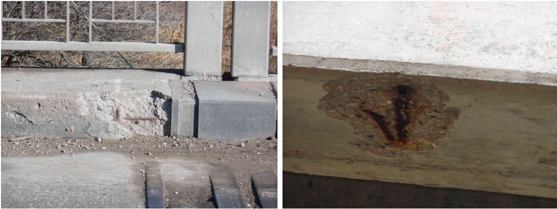
Figure 1.1: Example photos of spalls. (Photos by: Region of Waterloo)
