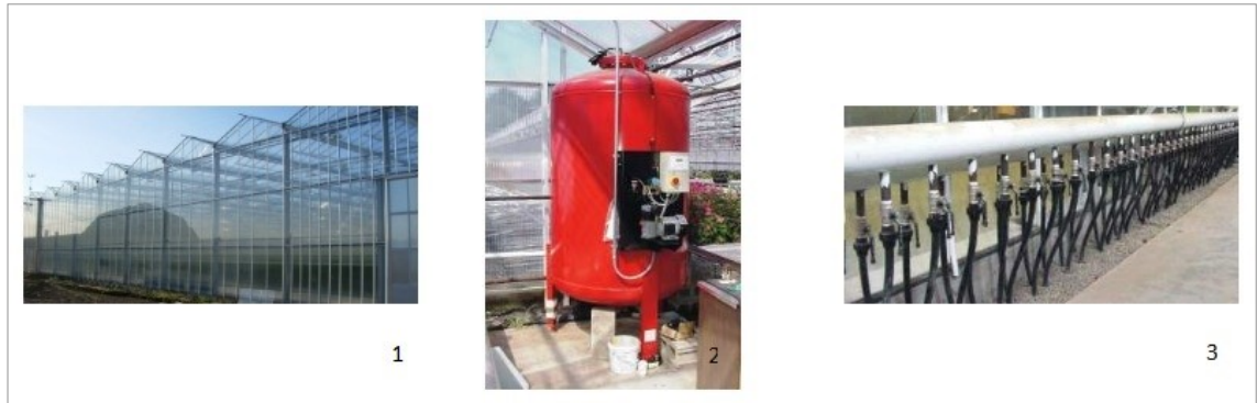
Figure 25. Greenhouse at Westland, Netherlands (1. Venlo-type greenhouse, 2. Pressurised hot water boiler, 3. Heating mechanism) (Venlo AP Holland Group, no date)
