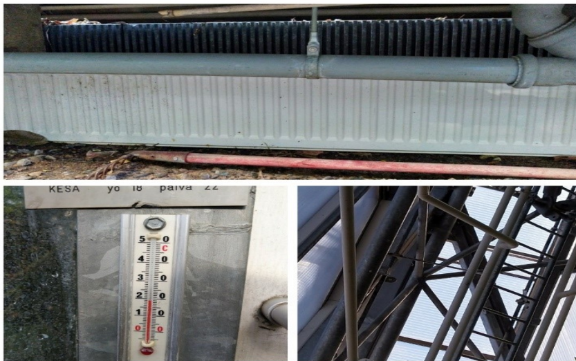
Figure 31. Radiator heating systems in the greenhouse
