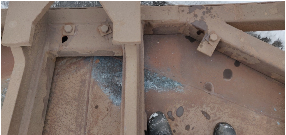
Figure 33. Large area has been exposed to the heat for a relatively short duration.
