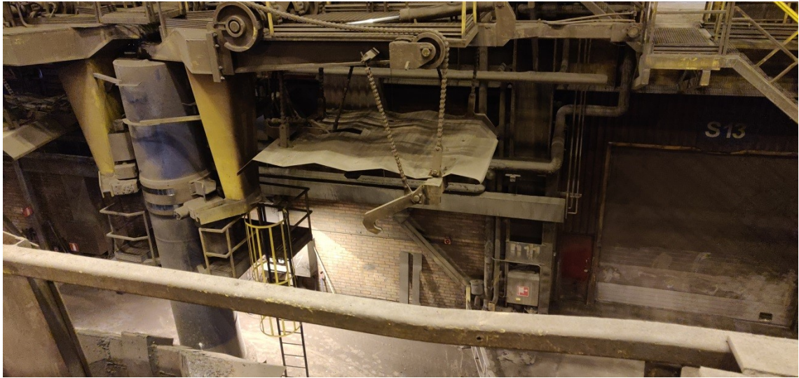
Figure 14. Lid storing system at ladle furnace.
