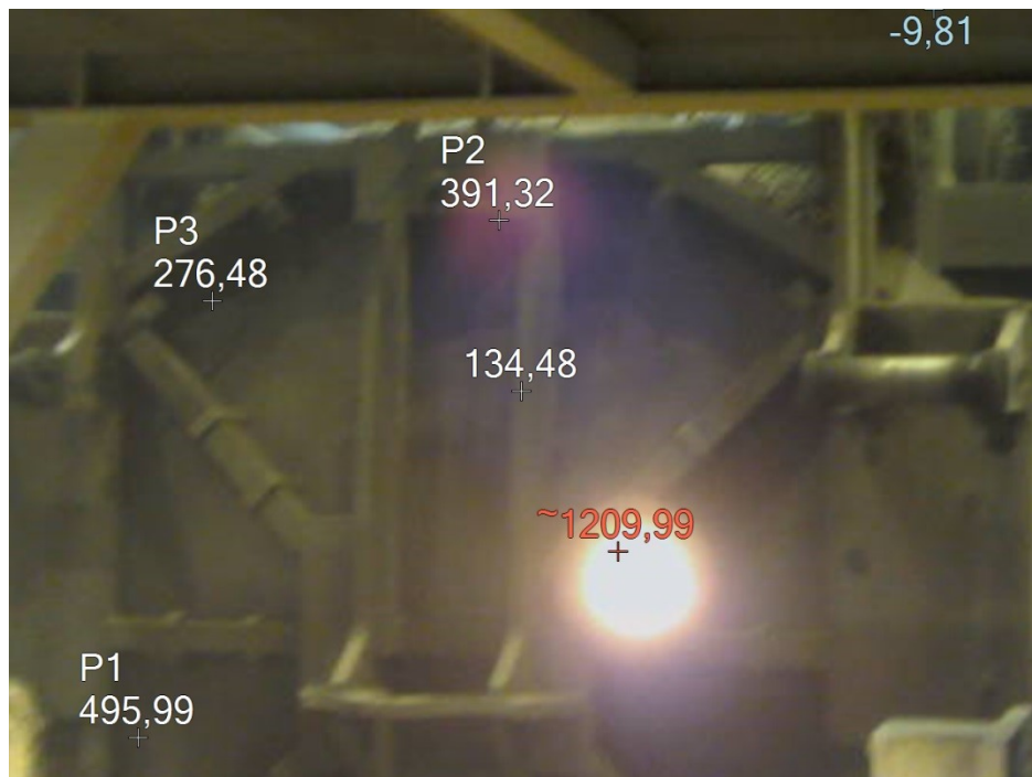
Figure 47. Visually, the backplate seems to be in decent condition.
