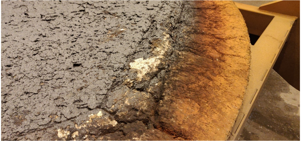
Figure 42. Fractures become deeper as time goes on.
