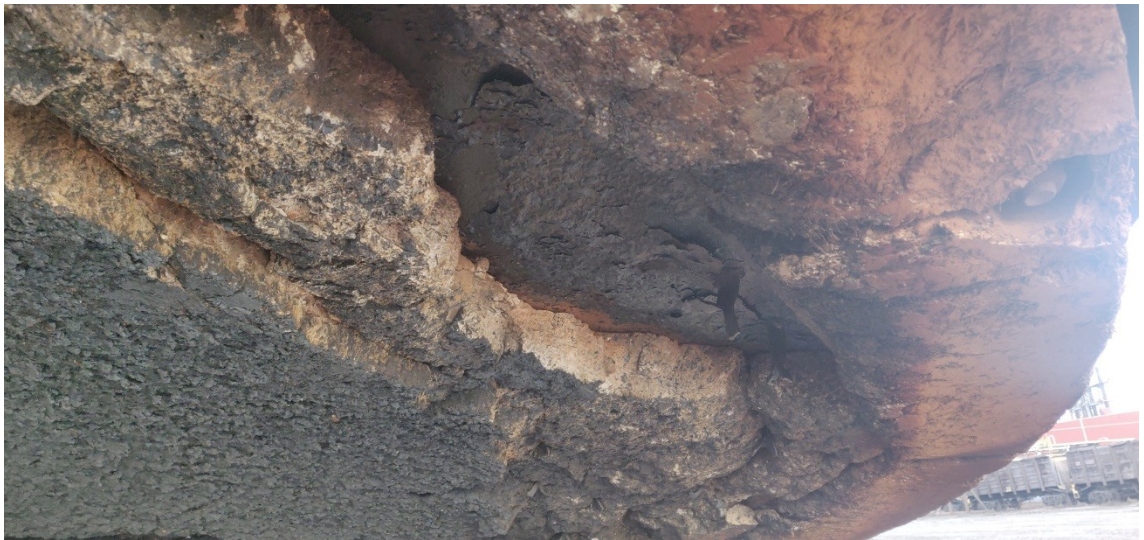
Figure 36. Heat has corroded most of the anchors and severely damaged the plate.
