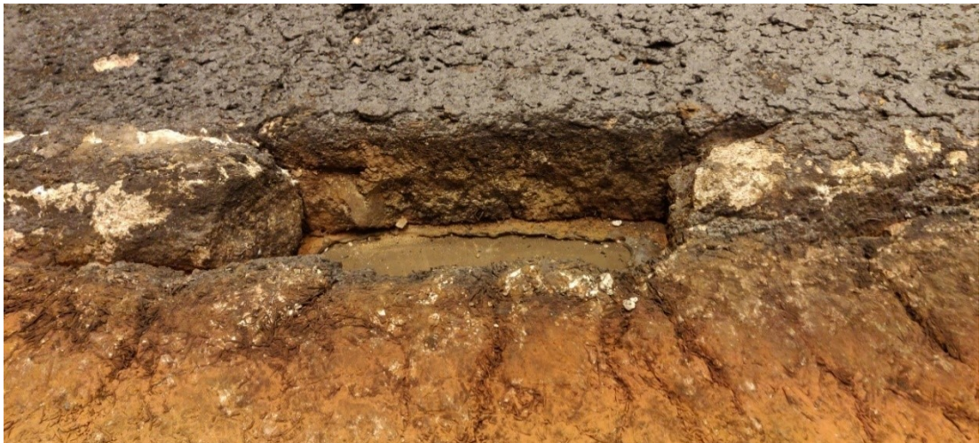
Figure 43. Large piece of refractory has fallen off exposing the metal cover.
