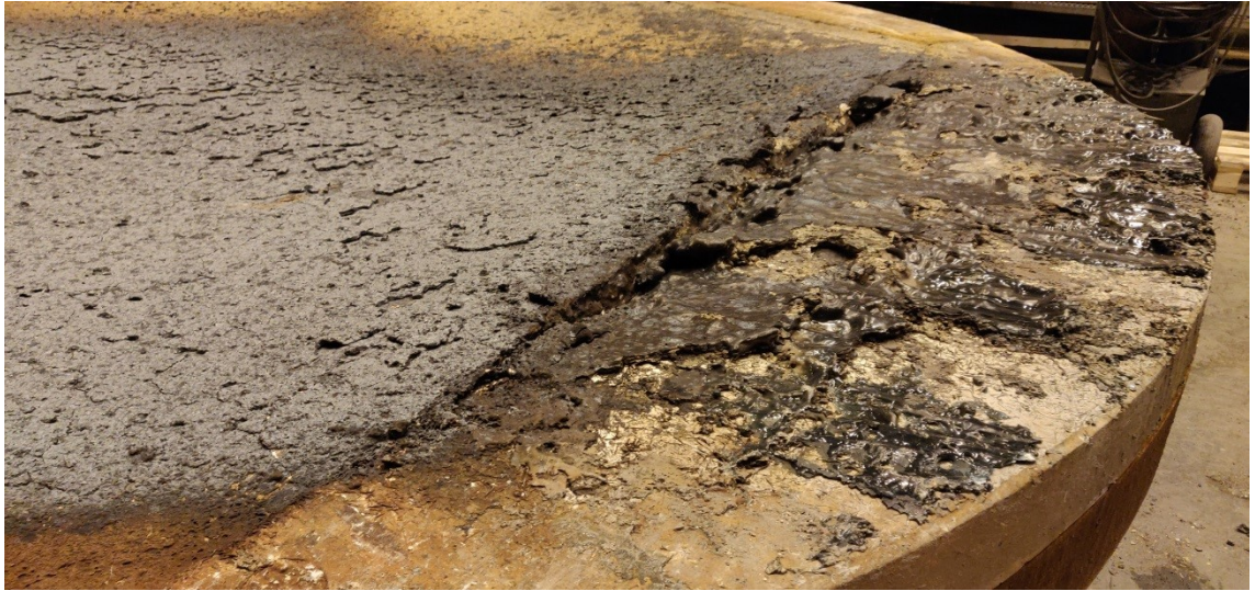
Figure 40. Condition of the peak brick after 200 heats.
