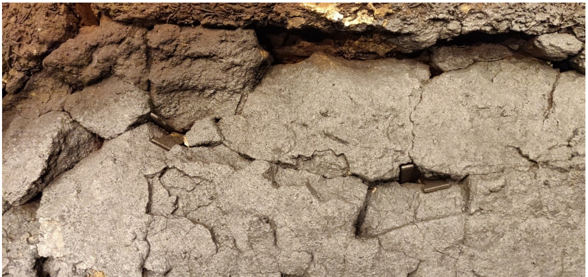
Figure 52. Metal anchoring seems to be in the focuses of the cracks.
