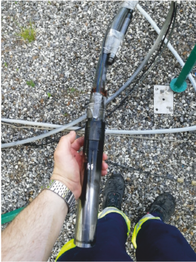
Figure 18. Overheated pump on the third pumping. The normal colour of the MP pump is metallic grey as in the lower parts of the pump. The black contamination on the picture is a mix of iron sulphide and soot. The figure also shows the pressure probe above the MP pump, which measures the hydraulic head inside the pump container.
