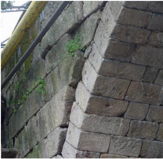
a) Sliding of the spandrel wall over the arch barrel.
