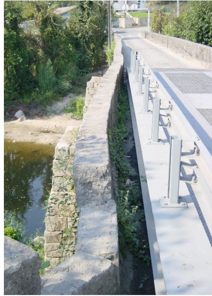
b) Out-of-plane deflection of the spandrel wall.
