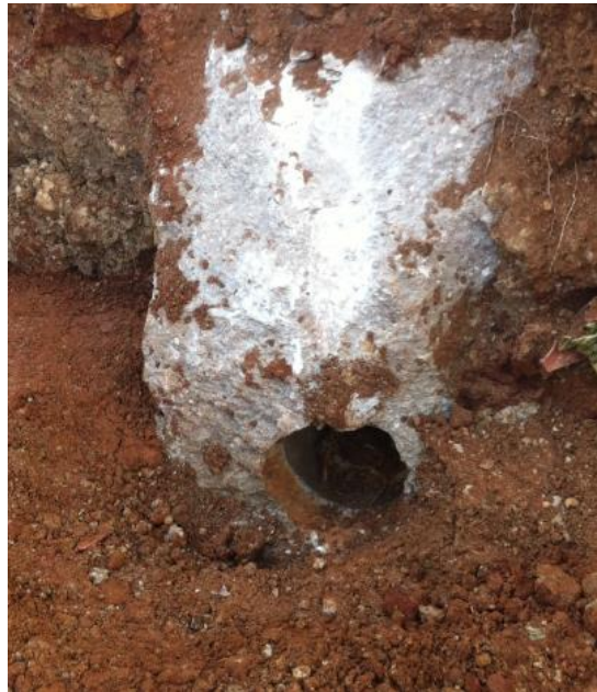
Figure 89: Rainwater drain line on the edge of the plot
