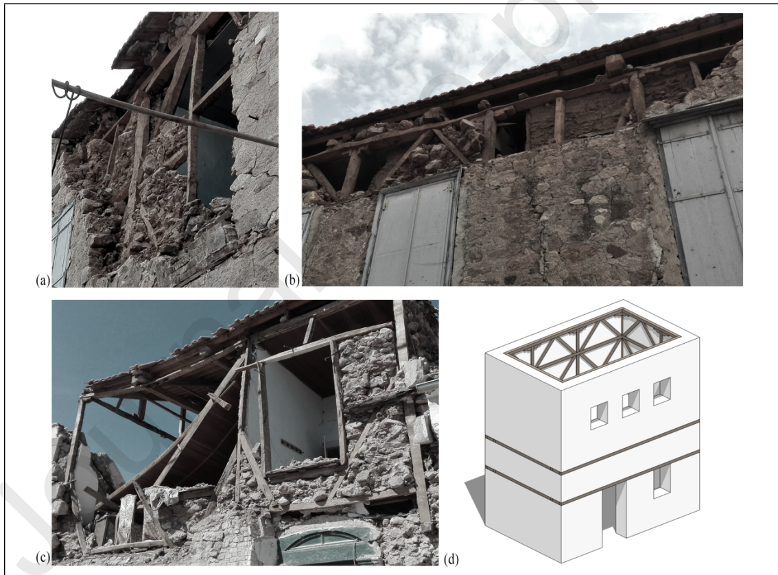
Figure 7. (a)-(b) Localized out-of-plane collapse of external unreinforced leaf. Notice the L-shaped corner elements in (b). (c) Extensive damage due to timber deterioration and poor connections. Notice the lack of the timber-frame system at the ground floor. (d) Schematic sketch of timber-frame masonry.
