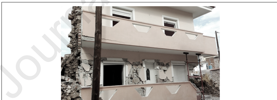
Figure 21. Severe in-plane shear damage at the ground floor of a building with large mass in the reinforced concrete floor slabs.
