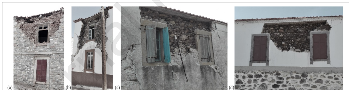
Figure 8. (a)-(d) Local failures of the external leaf due to wall disintegration.
