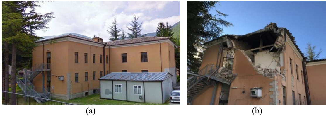
Figure 7: The corner mechanism activated in a masonry building during the 2016 Central Italy earthquake.
