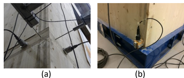
Figure 6. Accelerometers installed on the building. (a) Method used in the 1 st and 2 nd floor; (b) Method used on the ground floor
