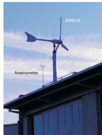
Figure 1. Small-wind generator of 3.5 kW analyzed.
