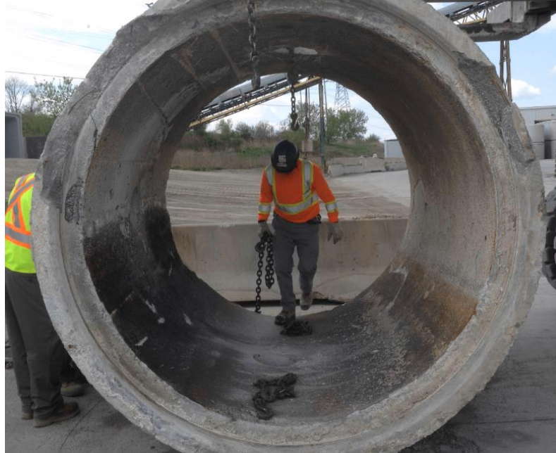
Figure 2: A 40-year-old concrete pipe showing the level of sewage.
