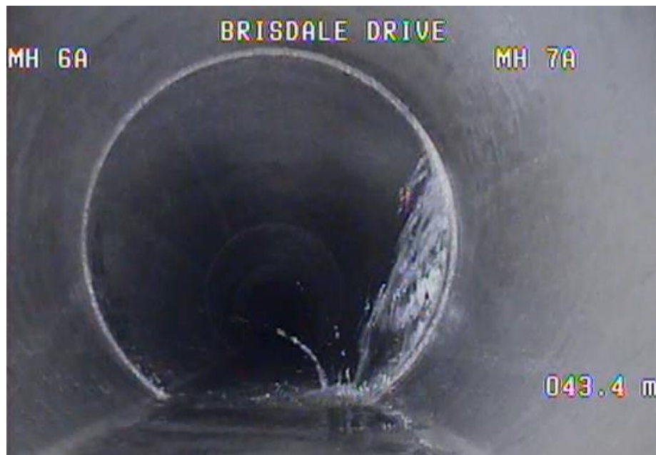
Figure 1: CCTV showing Type 3 Infiltration as per ASTM C1840 (2017).
