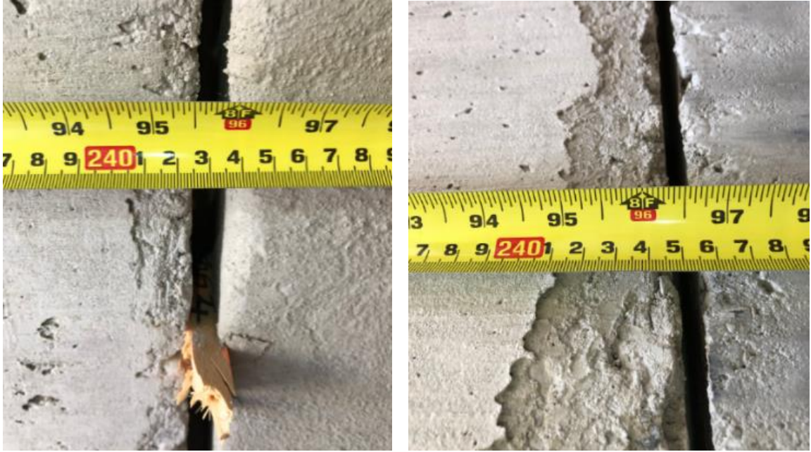
Figure 38: Joint gap on the (a) left, and (b) right side of the pipe created in the job site to account for the manufacturing tolerance to maintain sewer alignment.
