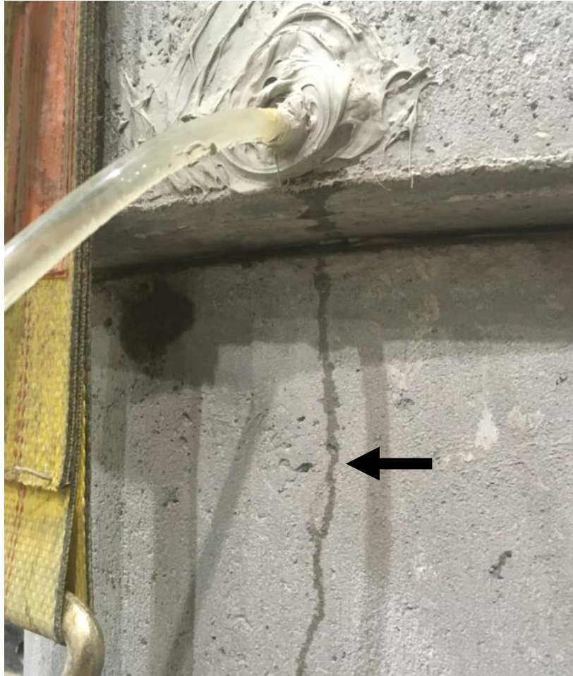
Figure 30: Leakage from Inlet Tube Caulking (600mm at 300 kPa).
