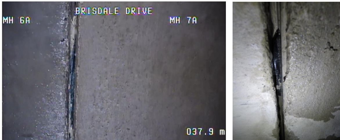
Figure 37: (a) Left: Displaced gasket captured by CCTV and (b) Right: observed in the infiltration test.
