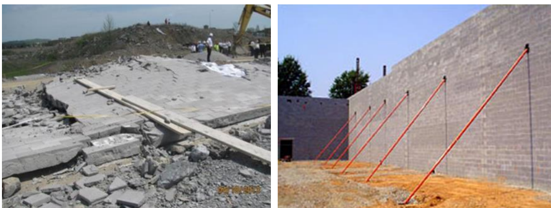
Figure 1.1: (a) Catastrophic failure of masonry wall (DOC 2013), (b) a temporary external bracing system during construction (Lang 2005).
