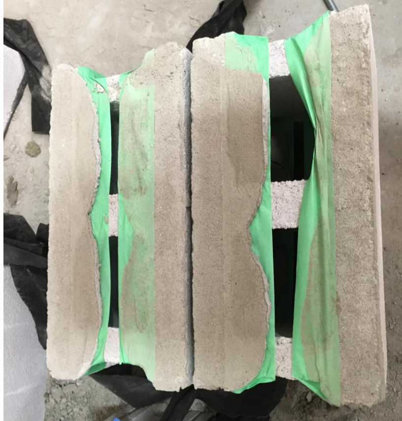
Figure 2.13: Typical de-bonding failure of early-age masonry.
