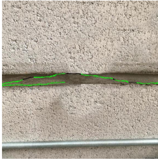
Figure 4.18: Pixel-level localization of early-age masonry crack.
