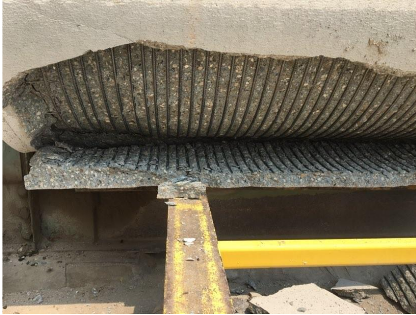
Figure 4.10-Concrete Slabbing Failure in RCP with SE Cage Reinforcement
