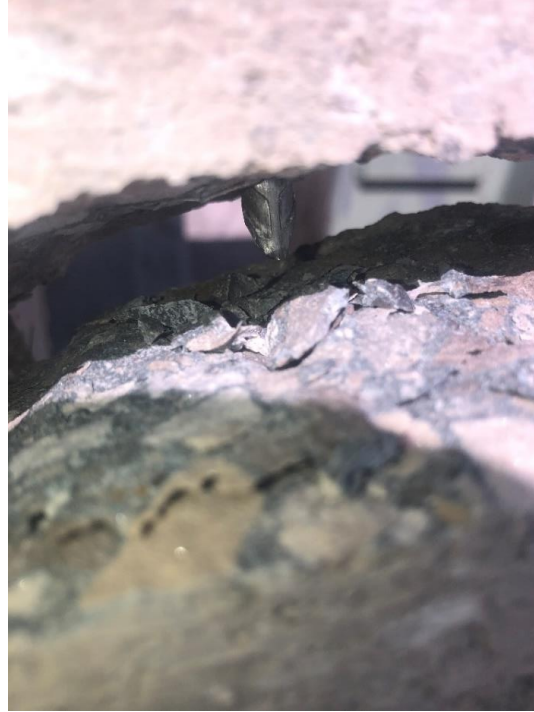
Figure 3.18-Evidence of Steel Fracture in DC RCP Specimen.
