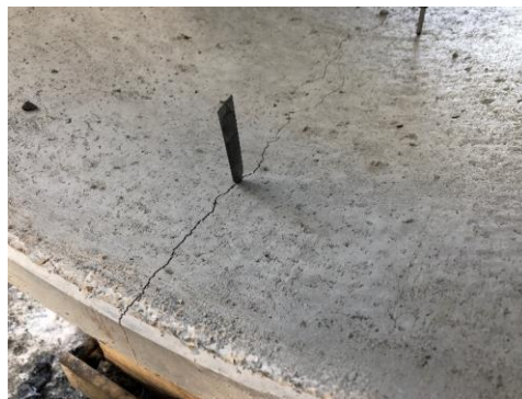
Figure 2.2-Leaf Gauge Measuring 0.3 mm Crack.
