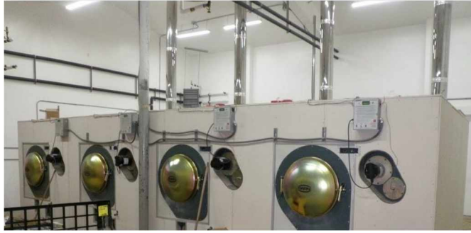
Figure 3.4. Biomass boilers use locally harvested wood resources for district heating in Tanana Alaska. Source: Alaska Center for Energy and Power, University of Alaska Fairbanks.
