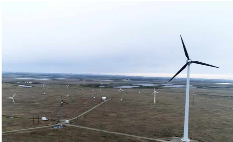
Figure 3.9. Kotzebue, Alaska has close to 3 MW of installed wind power, a 1.2 MW Li-ion battery, and dispatchable loads including thermal electric boilers, absorption chiller for ice-making, and an organic Rankine cycle generator. Source: Alaska Center for Energy and Power, University of Alaska Fairbanks.
