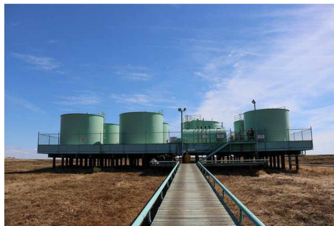
Figure 3.6. The Kongiganak, Alaska bulk fuel storage facility stores 1,317,200 liters (348,000 gallons) of diesel and gasoline. Source: Alaska Center for Energy and Power, University of Alaska Fairbanks.
