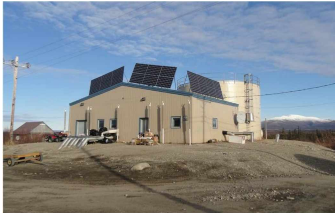
Figure 3.5. A 10 kW solar PV array installation on the water treatment facility in Shungnak, Alaska in the Northwest Arctic Borough. Source: Rob Bensen, Bering Straits Development Corporation.
