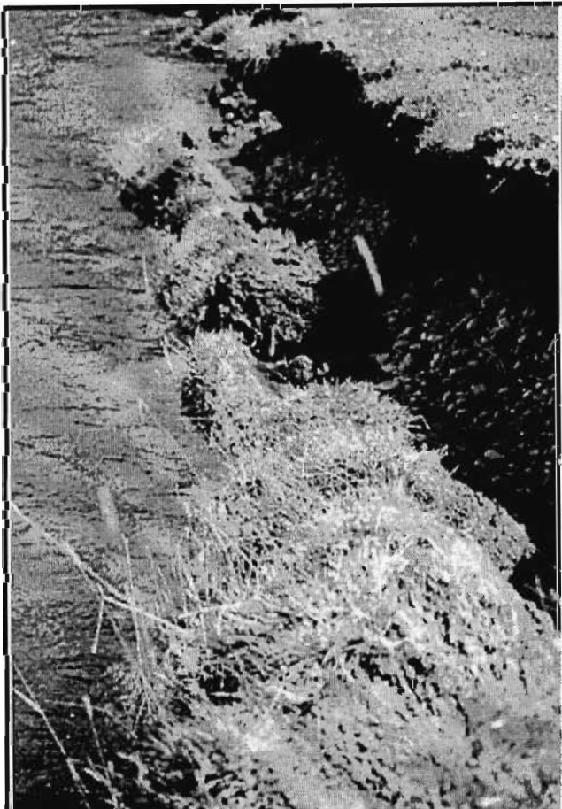
d) cantilever failure : the collapse of an overhanging block into the channel.
