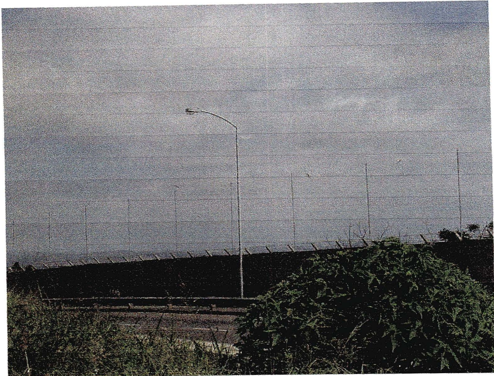
Plate 7: New odour control fenceline misting system
