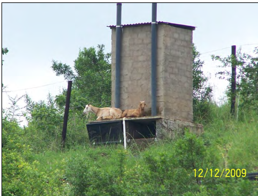
Plate 6.2: Twin vault UDD Vault Latrines
