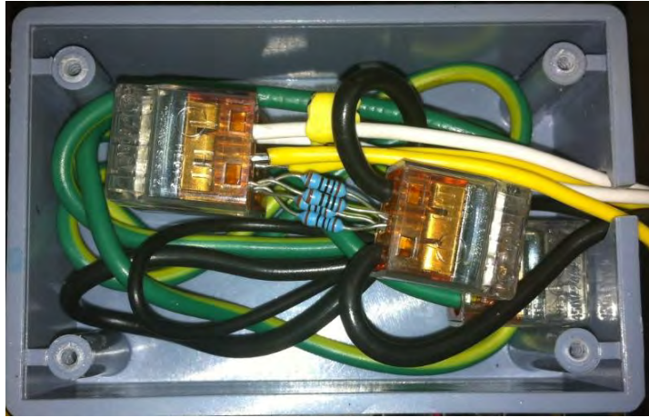
Figure E.3 Pull down resistor of 10\text{ k}\Omega grounds floating signals present in PWM.
