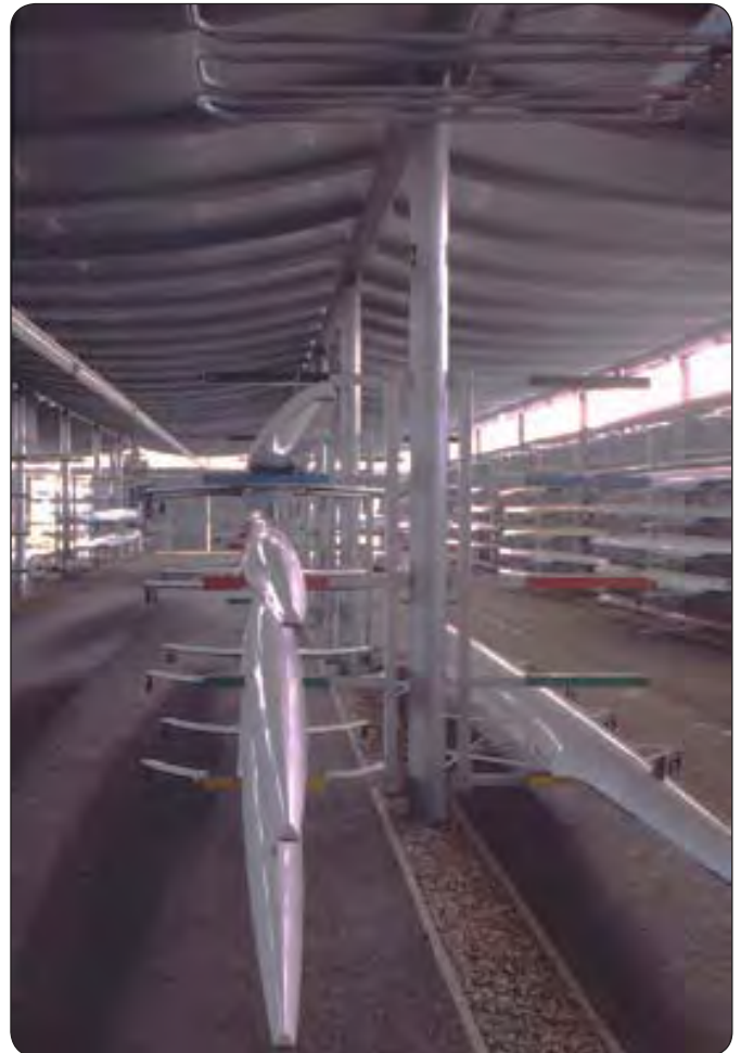
Illustration 04.70: Interior view of the boathouse with gap between the gabion wall and roof allowing light and ventilation into the space.
