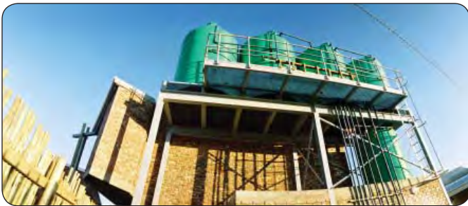
Illustration 03.17: Water storage tanks used at the Seven Fountains Primary School where a comprehensive network of gutters and water tanks collect the rainwater from roofs. This water is used for washing, and for watering the gardens and sports fields.
