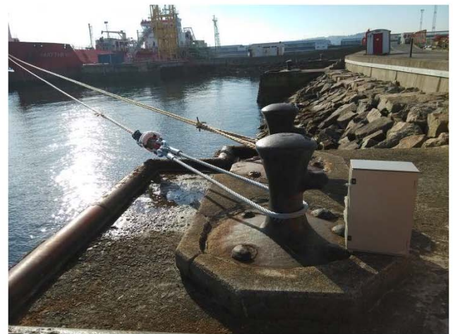
Figure 7. Load cell installed in the Inner Port of A Coruña (Spain).
