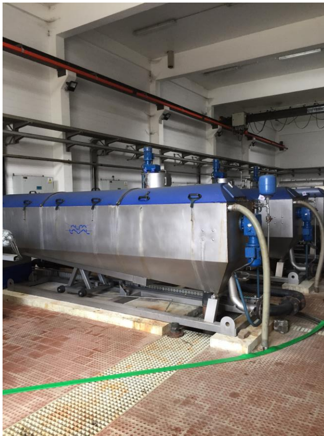
Mechanical thickeners (3) – receives biological sludge
