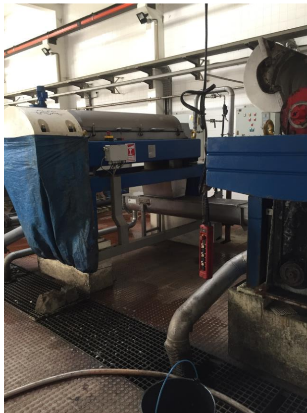
1 of 3 dewatering centrifuges
