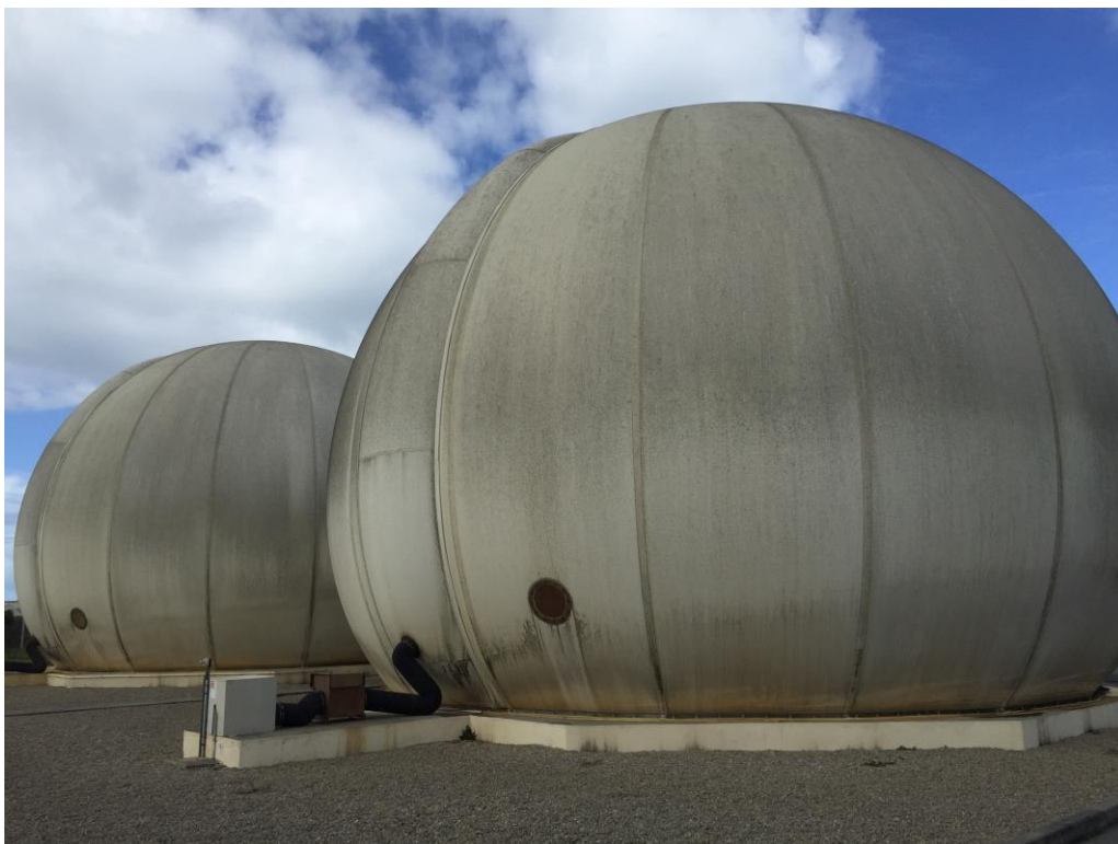
2 of 2 biogas holders
