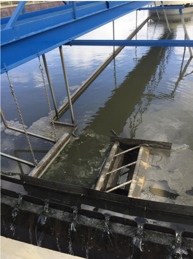
Secondary clarifier surface skimmer arm and trough for scum removal
