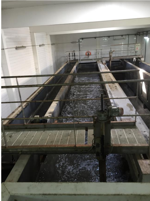
Aerated grit chamber
