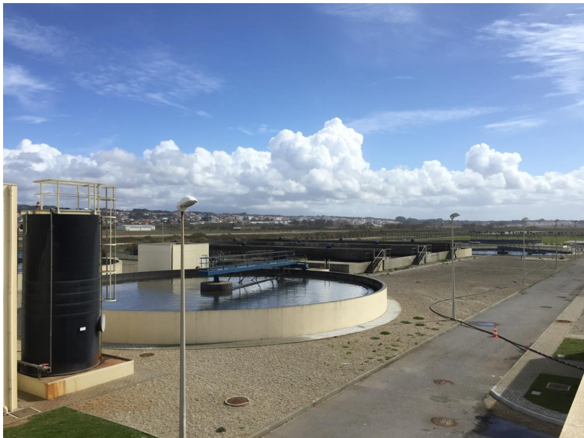
Figure 4.1-4: Espinho WWTP primary clarifier, biological reactor and secondary clarifier in the back. The black tank on the left is the PAX 18, the coagulant used in CEPT, storage unit.
