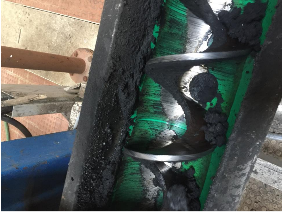
Dewatered sludge in the screw pump
