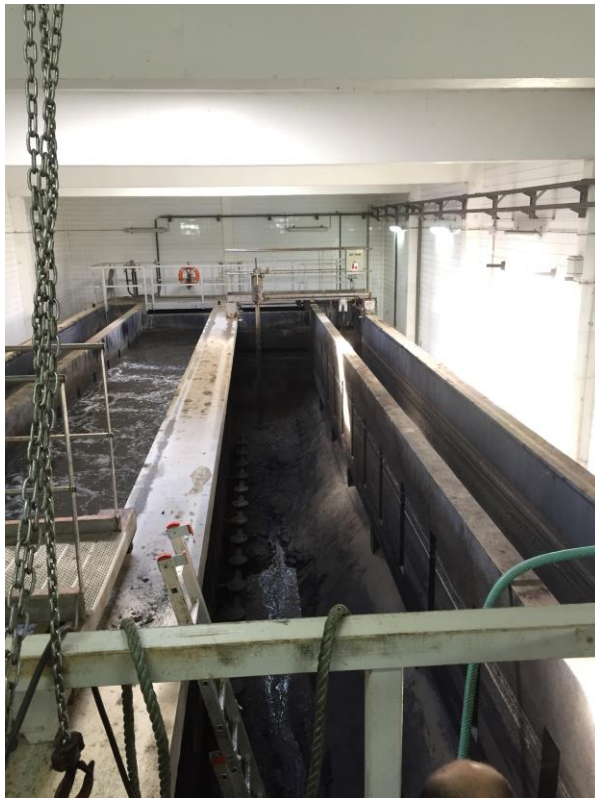
Empty aerated grit chamber (visible diffusers at the bottom of the tank)
