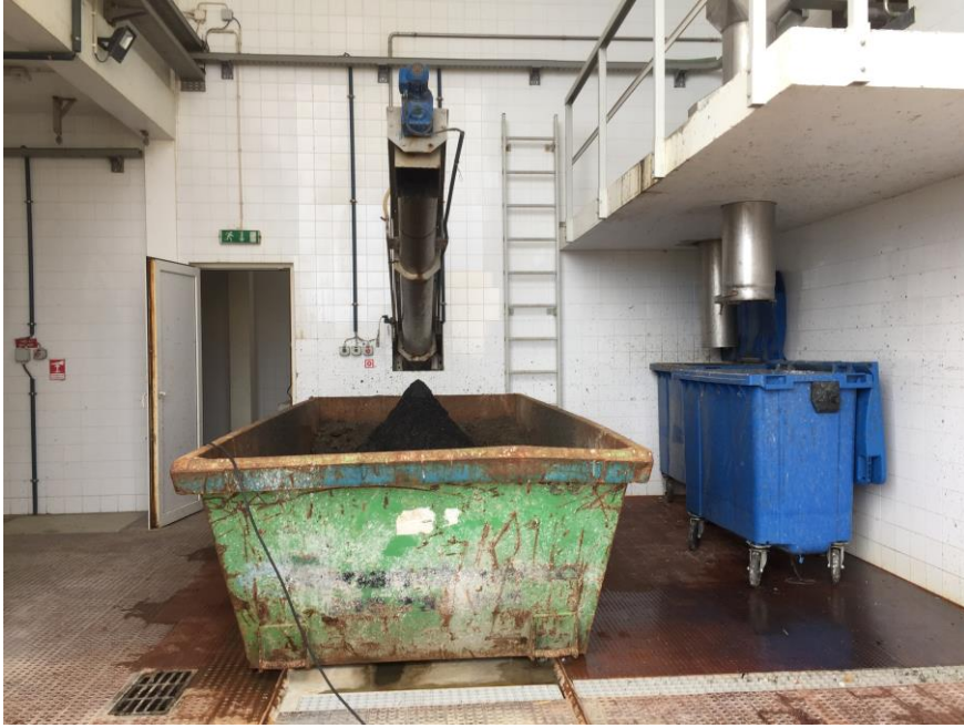
Grit storage container for disposal
