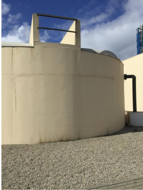
1 of 2 gravity thickeners – receives primary sludge
