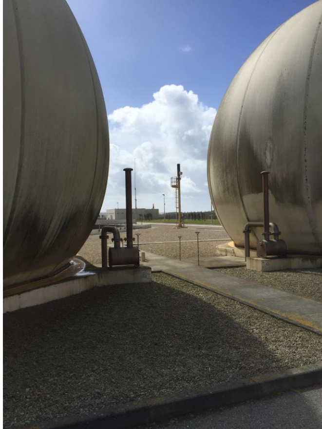
Biogas holders and biogas torch in the background (in the middle)
