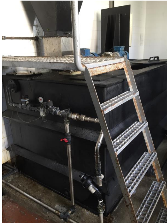
Polyelectrolyte preparation unit – for sludge conditioning of the dewatering and thickening processes
