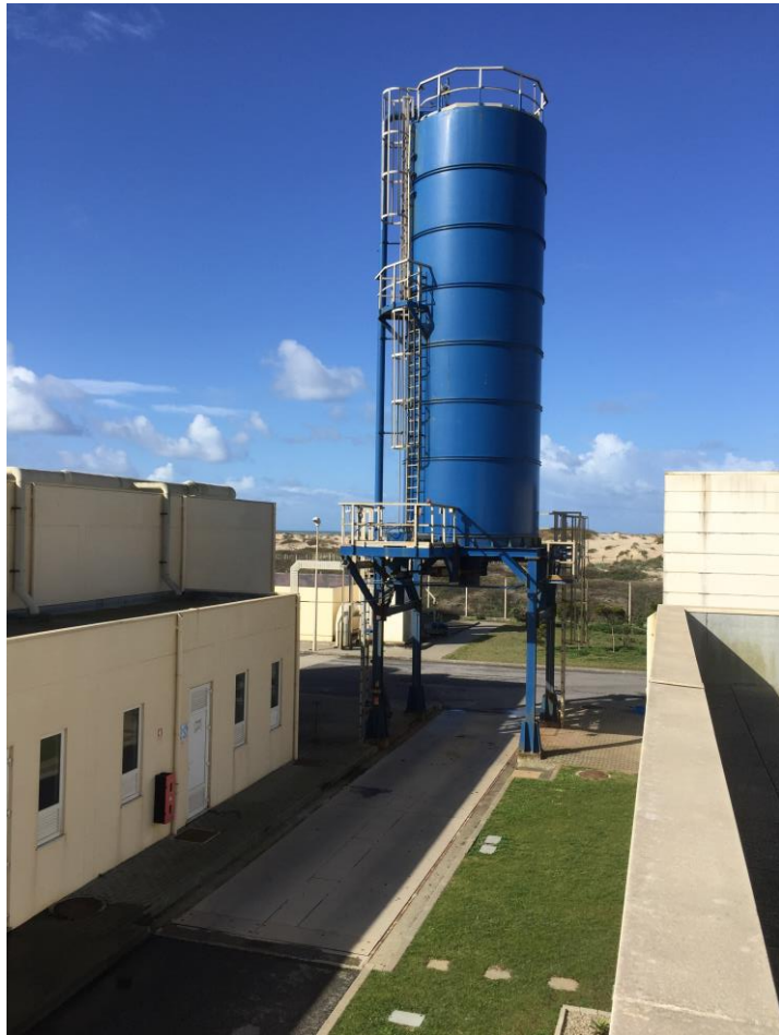
Dewatered sludge silo
