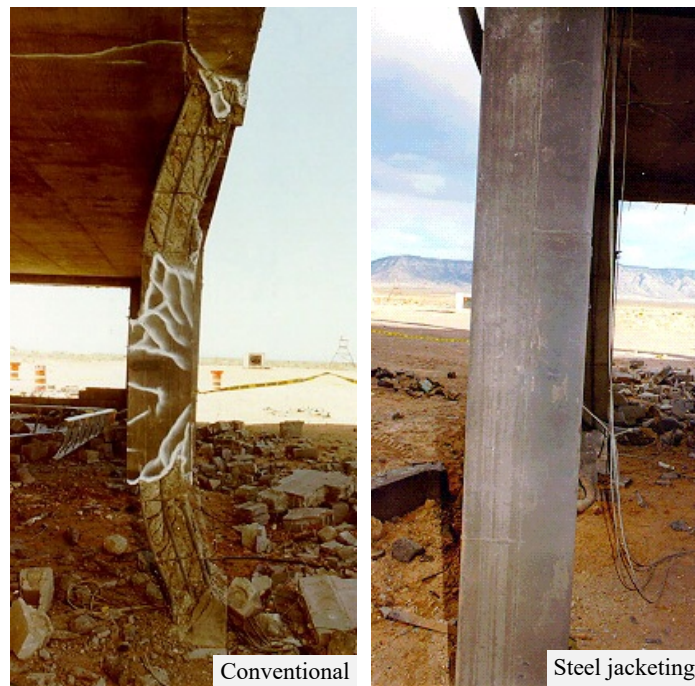
Figure 3.1: Enhancement of blast resistance of RC column by means of steel jacketing (Adapted from [103])
