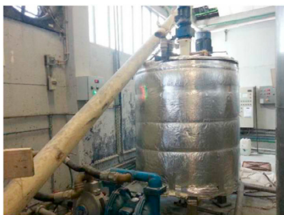
Fig. 13. Starch glue storage silo.
