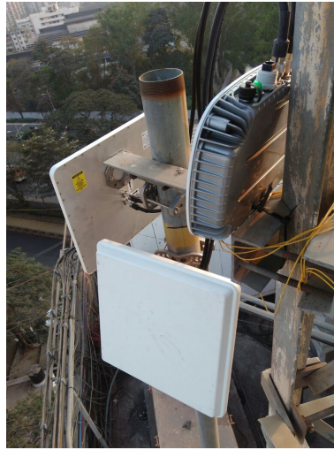
Figure 2.1: Example of a WiBACK node wrongly placed (connectors are facing upward and the water will leak over time).
